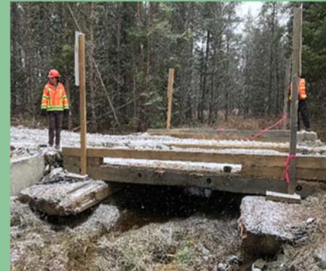
The field audit observed numerous examples of well-designed and installed (and removed) temporary bridges that effectively protected streams and streambanks (Licence 7).
