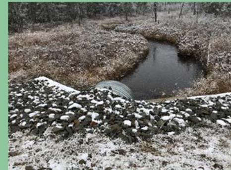
An example of a recently installed embedded culvert used to facilitate fish passage that replaced an old, failing pipe identified under the Company's road inspection and maintenance program (License 7).
